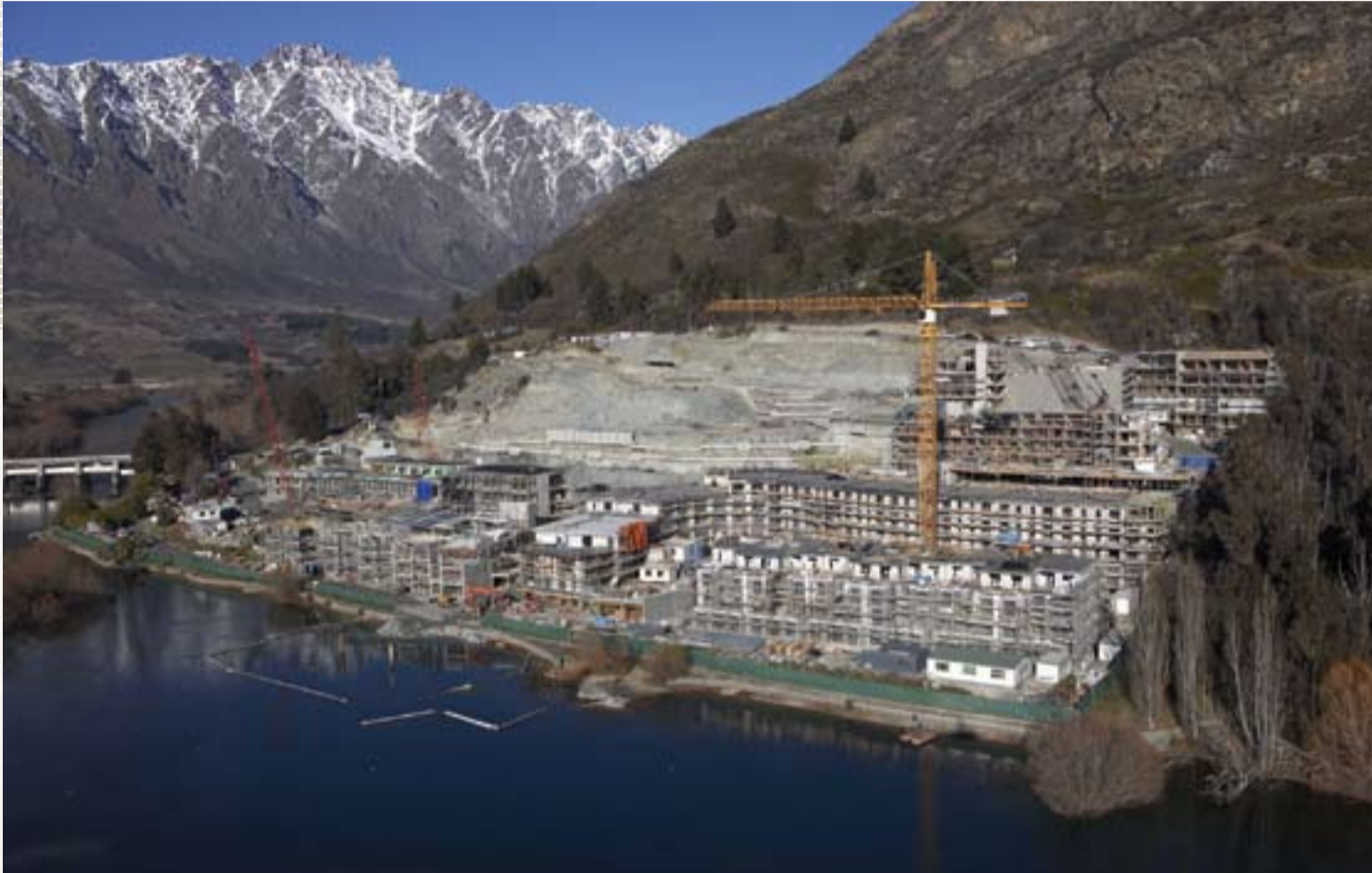
McConnell Property is providing development management services for Stage One of the Kawarau Falls Station Resort in Queenstown - 5 star and 4 star hotels with additional townhouses and luxury apartments.
