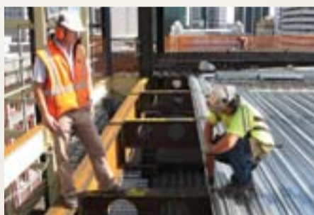
Warren Wilks (Hawkins) and William King (Composite Floor Decks) using suspended nets below as a means of 'isolating' the fall hazard.
